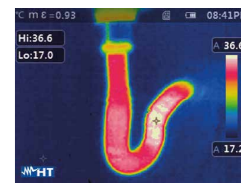
In the photo: thermogram of a clogged siphon acquired with THT80.
